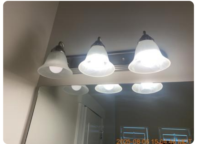
Light Fixture 2025-08-06 15:04:46 40.42173932175136, -111.8643382524245 View Image
